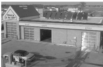
The solar thermal system installed on the Bonduel Car Wash in Bonduel, WI, saves the owners a substantial amount on their energy bill. The solar thermal panels heat water for washing vehicles and for the radiant floor heating system.
