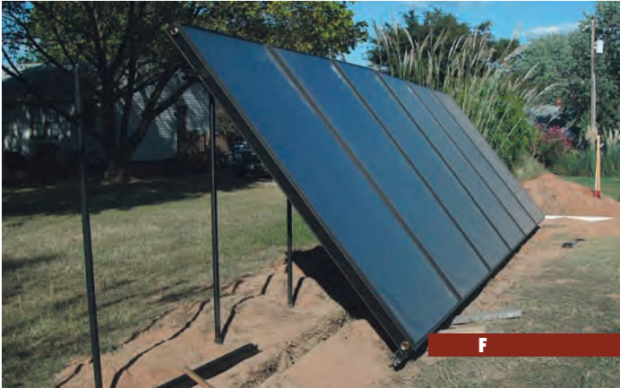
F, G - The authors installed the solar panel ground mounts in one day, dug in a few hours with a power auger. They spent another day trenching 2 feet deep under the mounts, for piping to the heatstore. The eight solar thermal panels were ground-mounted the next weekend.
